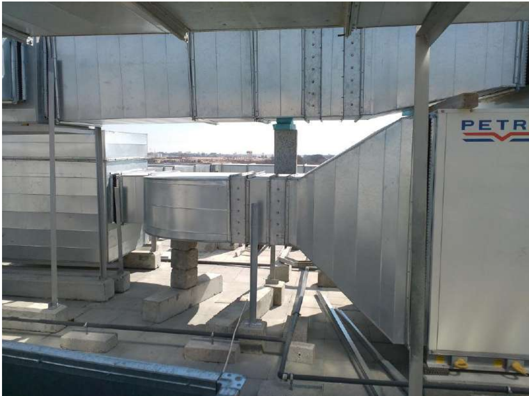
Waste Management Facility @ Ras Laffan (QP-5)
